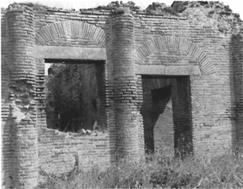
412 Openings at the Central Baths at Pompeii (62–79) overlaid by a lintel of tufa and relieved by a discharging arch.
