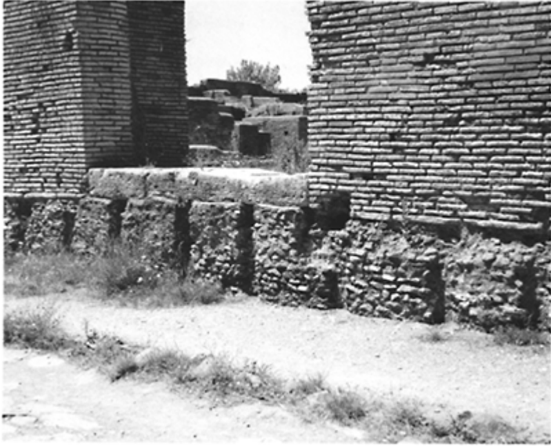
289 Foundations of the Casa dei Dipinti at Ostia, showing the imprints of the uprights of the framework (third century) used for buildings with walls of masonry or for ashlar construction.
