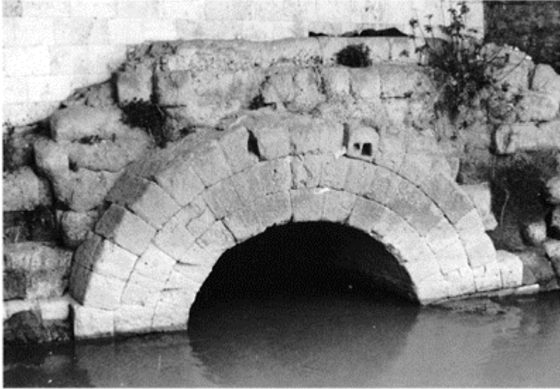
377 The outflow of the Cloaca Maxima into the Tiber, at the level of the Forum Boarium . The crown of the arch is made up of three rows of short voussoirs. The date of its construction is estimated to be the beginning of the first century BC.
