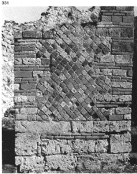
331 Complex opus mixtum , with a reticulate facing on a foundation of limestone blocks and quoins of block and brick. Pompeii VI, 3, 17.
