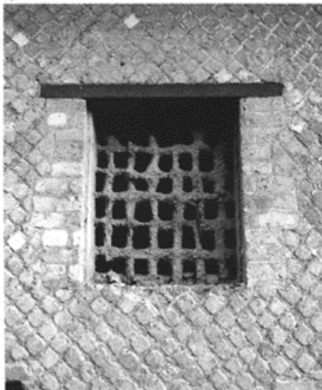
701 When ground-floor windows were of some size they were barred with an iron grille. This example is on the cardo IV, insula 5 , at Herculaneum.
