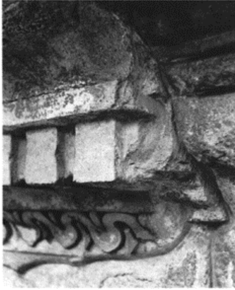
524 Detail from the cornice on the Temple of Portunus in Rome, showing the final moulding ( left ) in stucco (Lesbian cymatium, dentils, cyma) applied to a surface cut into the supporting tufa; c. 100BC.
