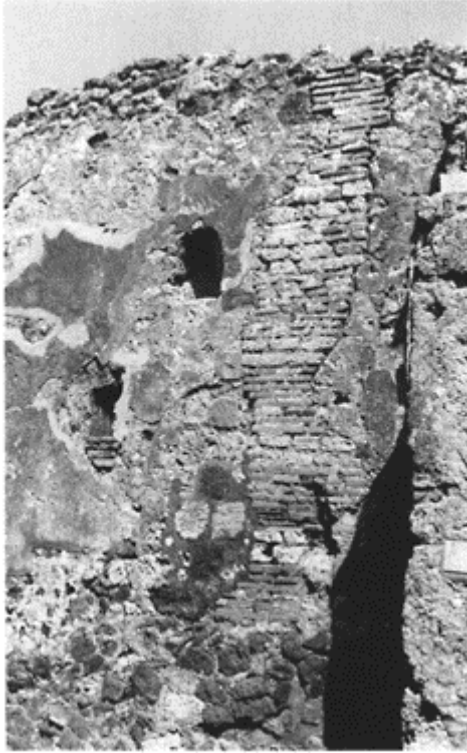
361 Pompeii, reconstruction after the earthquake of 62. A crack filled in with terracotta material and rubble (VI, 7, 5).
