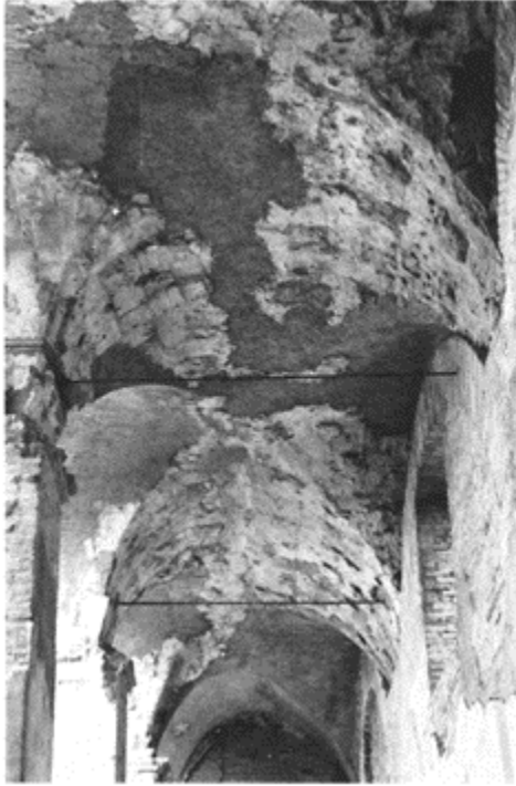
458 Rows of groined vaults made of masonry constructed on a permanent centring of square bricks. Ostia, House of Serapis.
