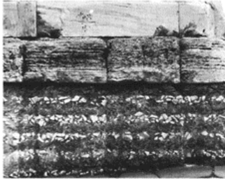
241 Foundations made out of coursed brickwork bearing traces of formwork, under the Arch of Titus; built by Domitian after AD 81.
