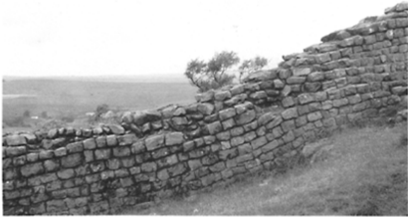
329 Section of Hadrian's Wall where the courses of the facing blocks follow the variations in the land surface (c. 128).
