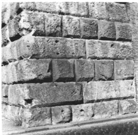
252 Regularly alternating courses of stretchers and headers on the aqua Claudia (38 to 52). The angled rustications (joints chamfered across their width) are coarsely scored. The whole takes on a great monumental
