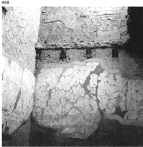
468 Remains of a floor and the beams supporting it in a house in Herculaneum.
