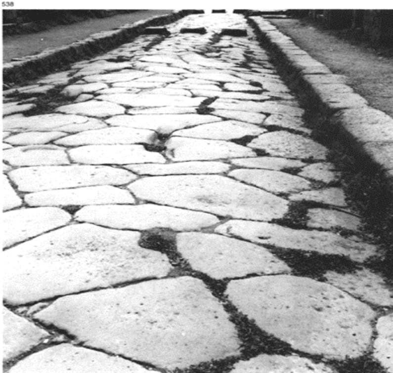
538 The paving of a commercial street in Pompeii, the via della Fortuna , of large slabs of lava, about 30cm thick.
