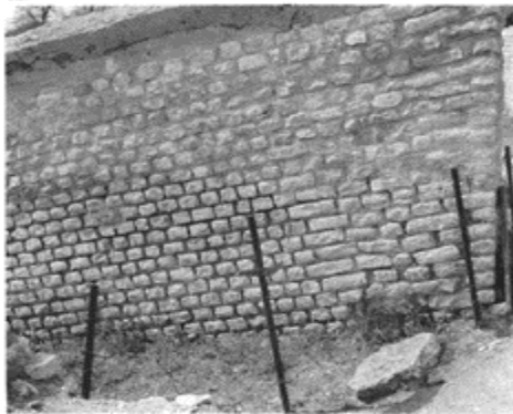
327 Internal wall of a vomitorium in the Gallo-Roman Theatre of Argentomagus, the courses of which follow the slope. First century.
