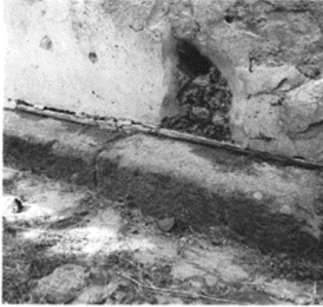
605 Lead piping from the temporary water supply network installed at Pompeii after 62. (VII, 12, 23.)
