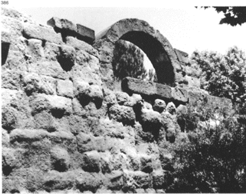
386 An opening for an artillery piece built into the Servian Wall, Rome around 90BC.
