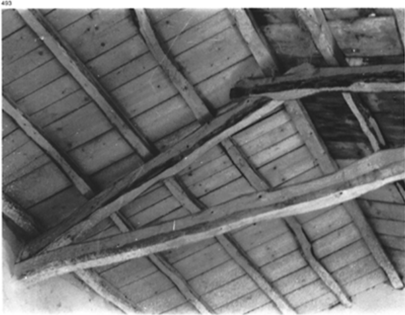
493 Roof timbers in a basic triangulated truss (one tie-beam, two principal rafters) supporting purlins and then boarding holding the tiles. The pieces of wood are not cut with a long saw but squared with an axe respecting the natural pattern of the grain. Roof of the Byzantine basilica of Aegosthenes (Porto Germeno, Attica). Span: 3.40m.
