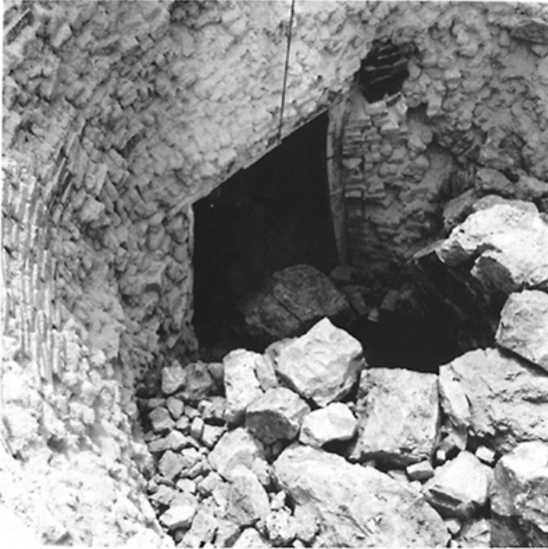
150 Construction and loading of the kiln at Foca (Campania); the combustion chamber is built up with the largest blocks.
