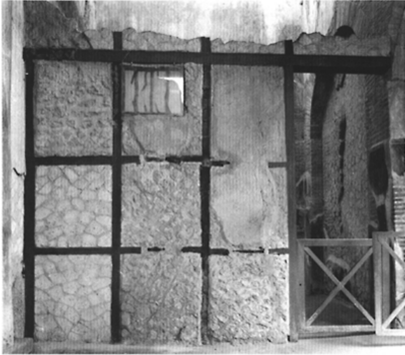
282 Herculaneum: timber—frame partition, opus craticium , built between 62 and 79 at the College of the Augustales. The infill is opus incertum and the whole was rendered. Thickness with rendering: 18cm. Section of the pieces of wood: 9×9cm.
