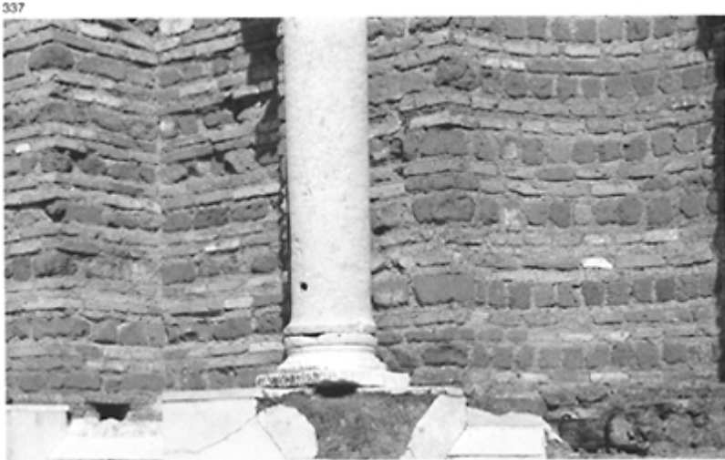
337 Ostia, House of Amor and Psyche, c. AD 300. Opus mixtum , alternating one course of blocks and two courses of bricks.
