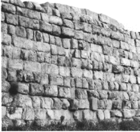
248 So-called 'Servian' Wall of Rome on the Viminal. Note the alternation of courses of stretchers and courses of headers; early fourth century BC.
