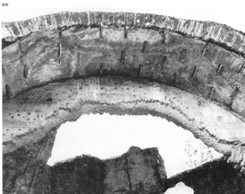
426 Marks of bricks placed straight on to the centring (which has collapsed) and ends of the radiating bricks visible in the intrados of the arch in the frigidarium of the Great Baths of Hadrian's Villa. Between 118 and 125.
