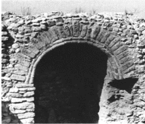
423 An arch on permanent coffering made up of a double row of ceramic cylinders. Baths at Sbeitla (Sufetula).
