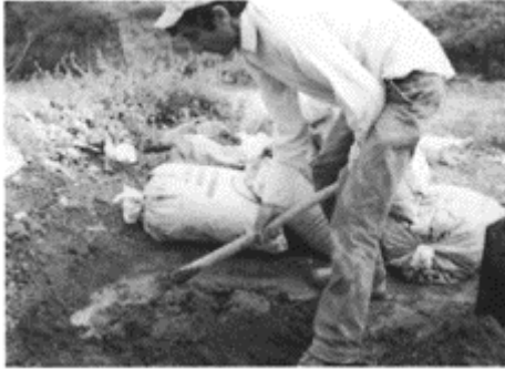
149 Clay being mixed for the repair of the interior surface of the kiln on the road to Epidaurus.
