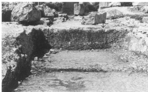
FIGURE 7.22. Temple of Apollo, foundation bedding for the south wall (arrows point to survey marks)
