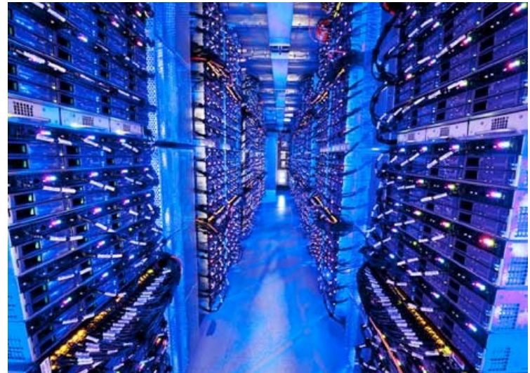
Inside a 40-ft Microsoft container, Chicago data center
